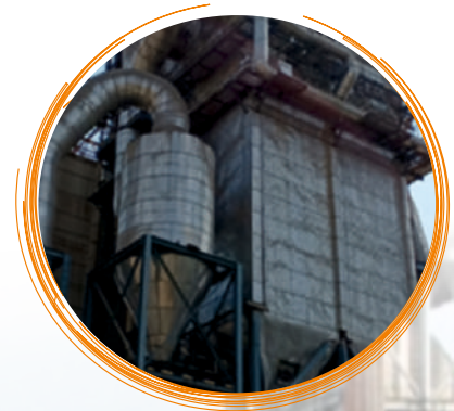
Vertical Cross Flow with Finned Tubes for AQC.
